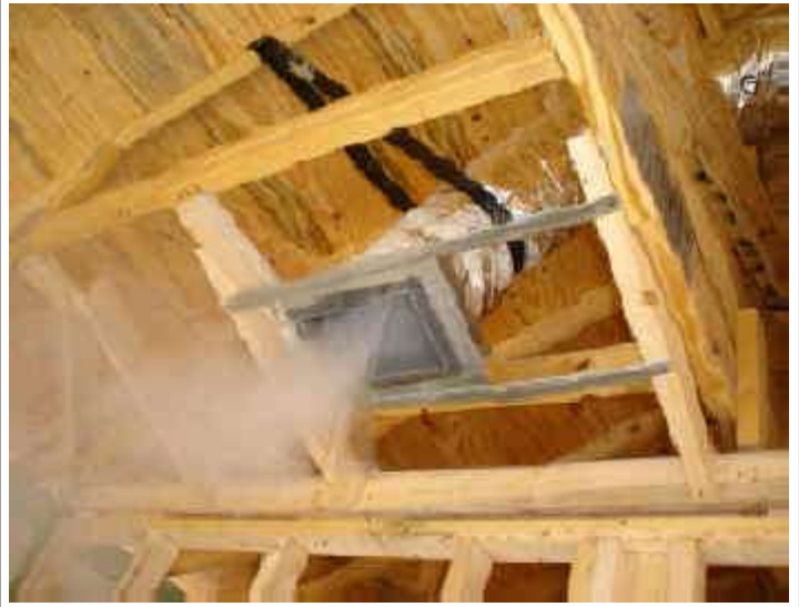
Most Remote register temporarily unsealed to allow fog to flow through entire Duct System
