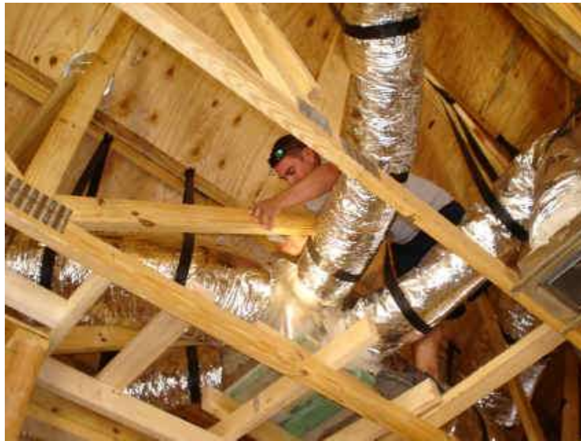
Duct Technician attending to leakage identified by smoke testing. Failures addressed now, will not be measured as leaks later, when it is too late or too difficult to correct them.
